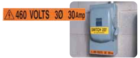
Electrical Panel ID
